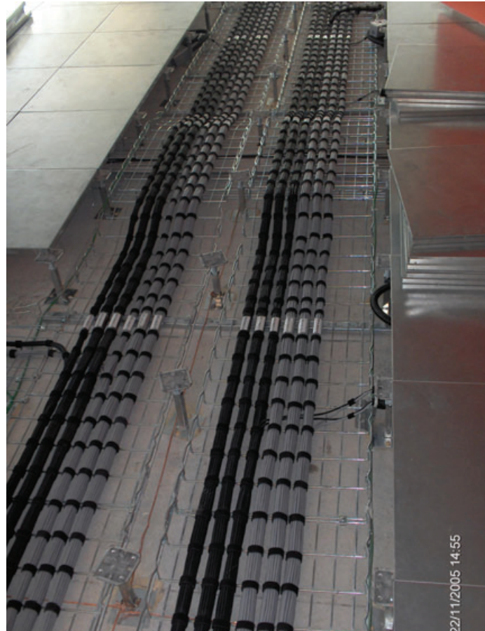
Figure 6: Structured cables under a raised floor
