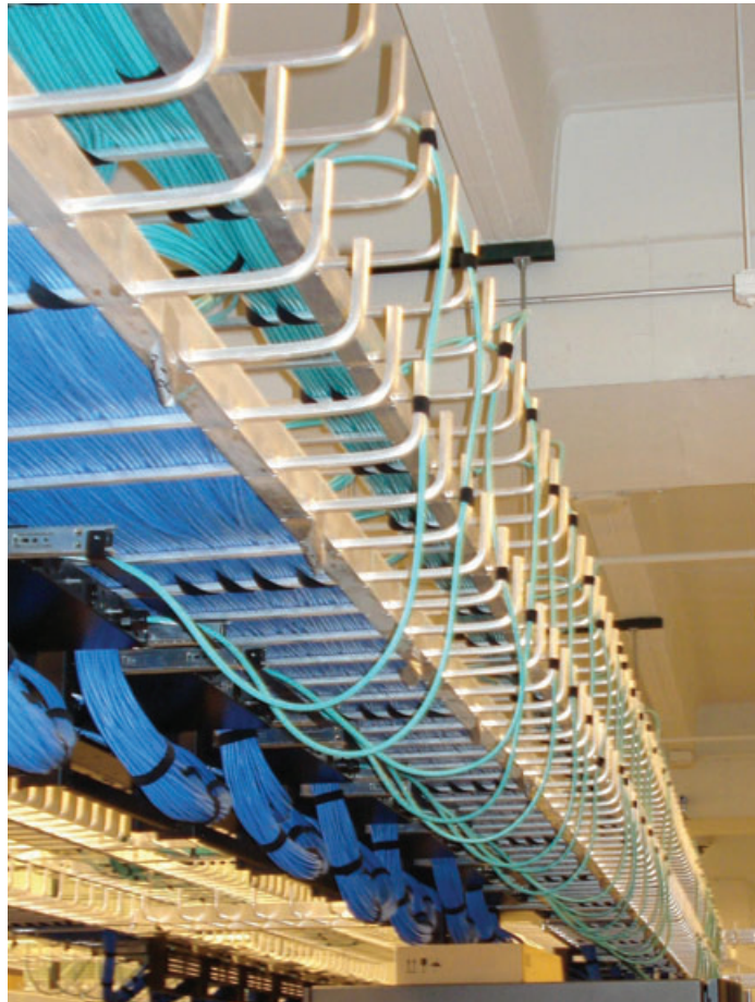
Figure 5: Structured cables in overhead space
