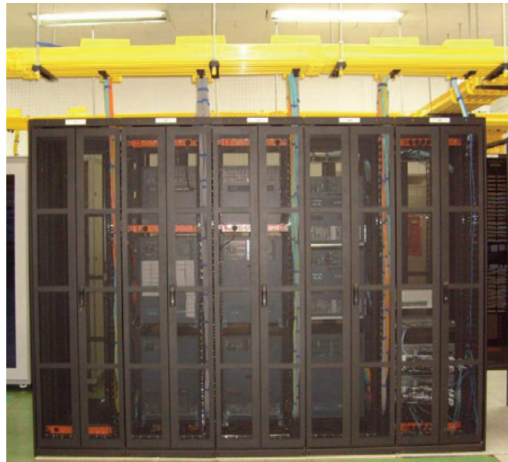
Figure 4: The HDA of a media company's Data Center
